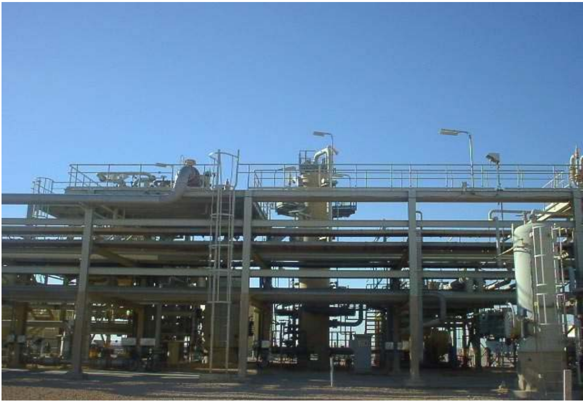
Salam Gas Plant (Khalda)
