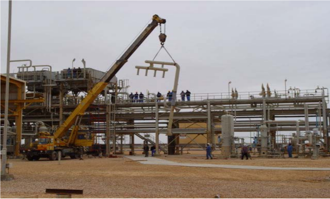
Tarek Gas Plant (Khalda)
