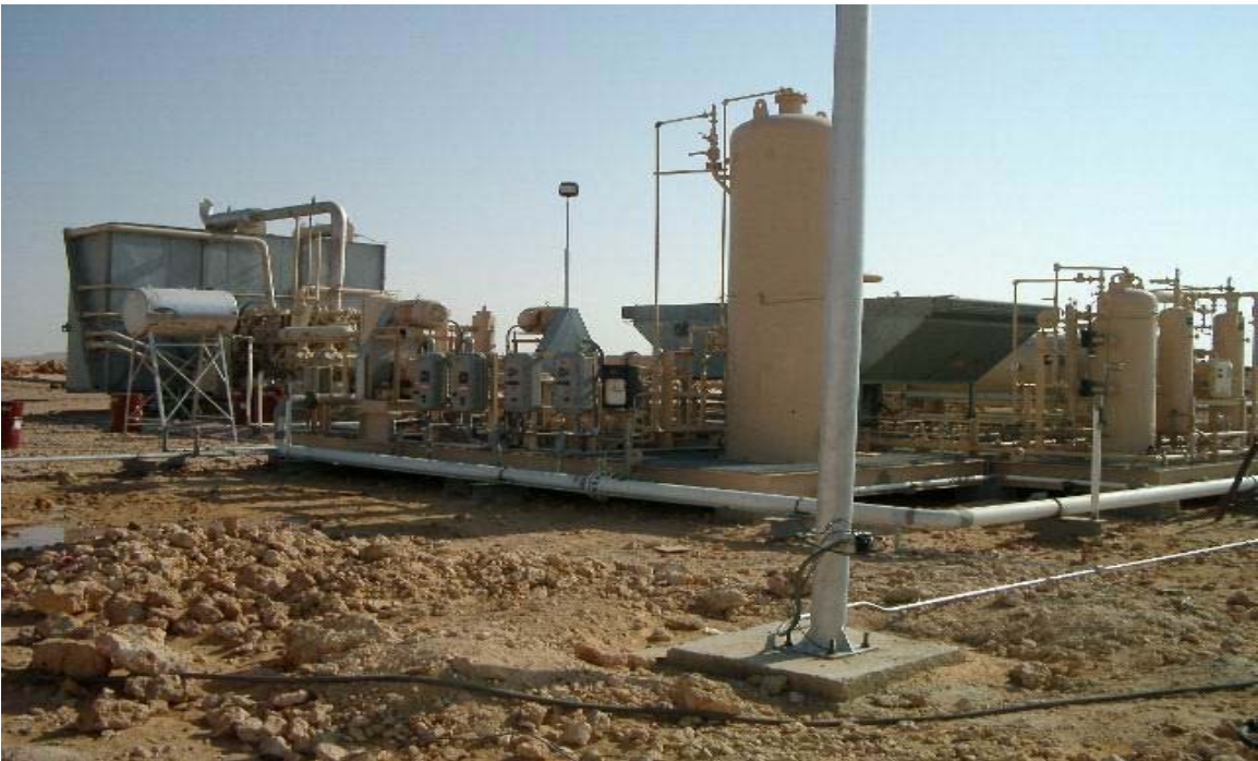
Nodal Compressor Station (Khalda)
