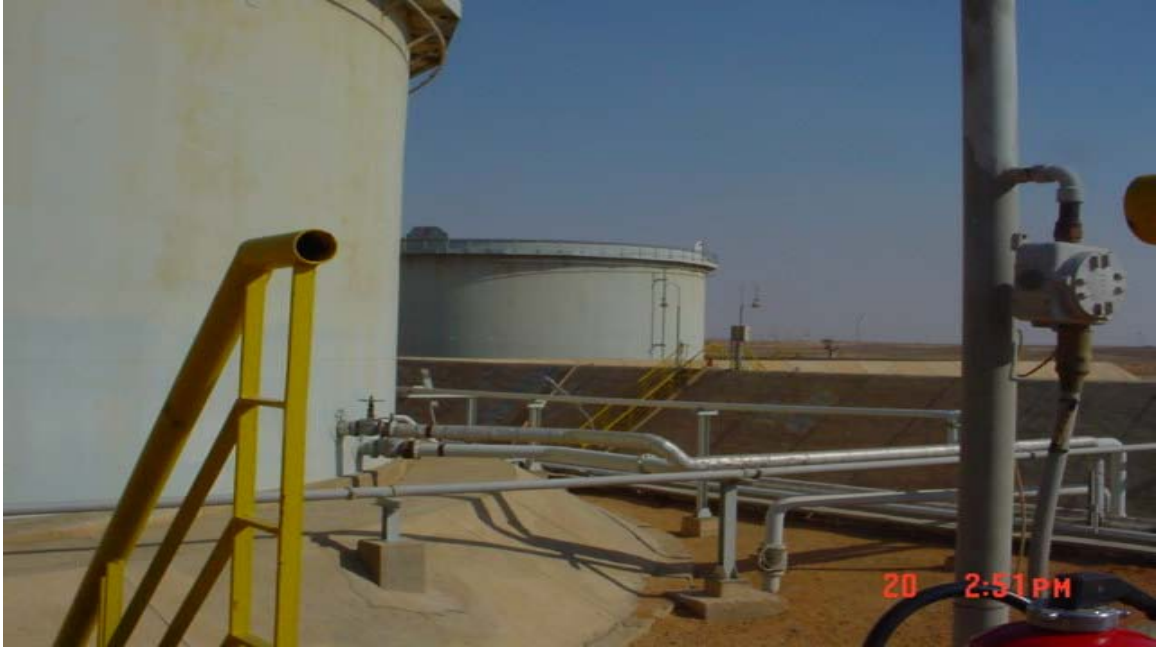
Tank Containment - Qarun Oil Process Facility
