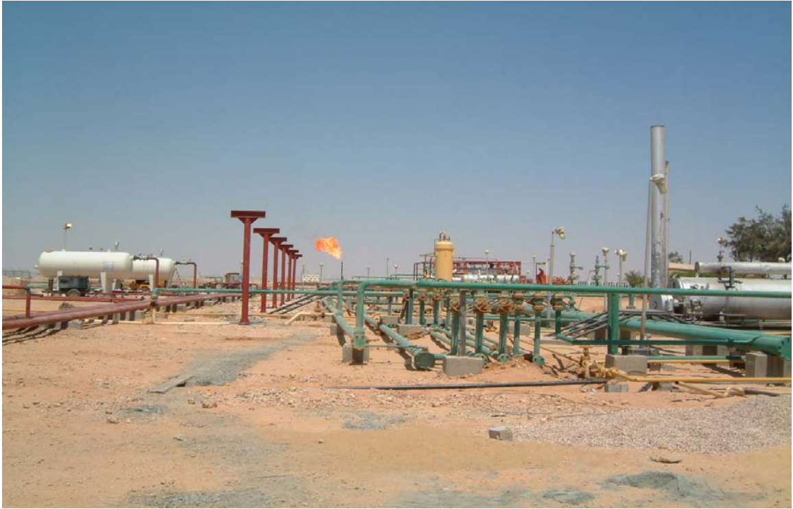
Umbarka Process Facility
