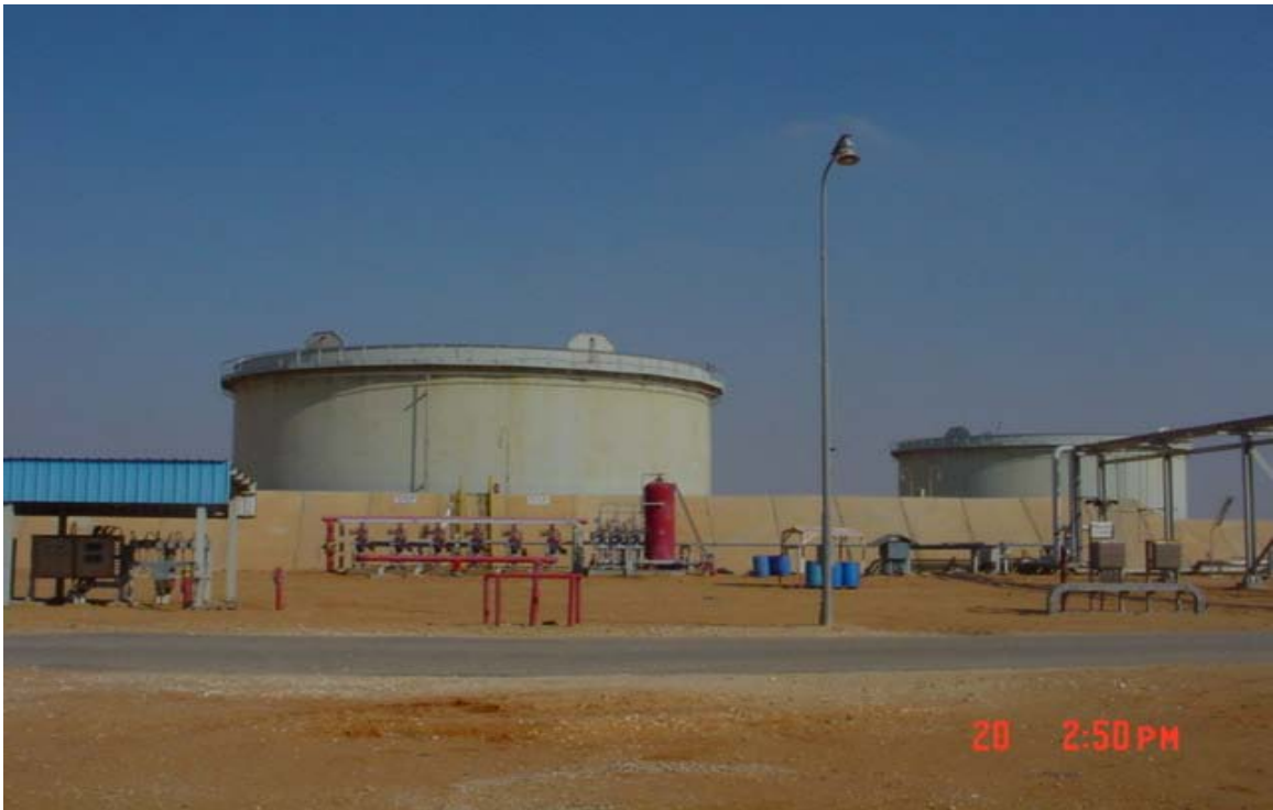
Storage Tanks – Qarun Oil Process Facility
