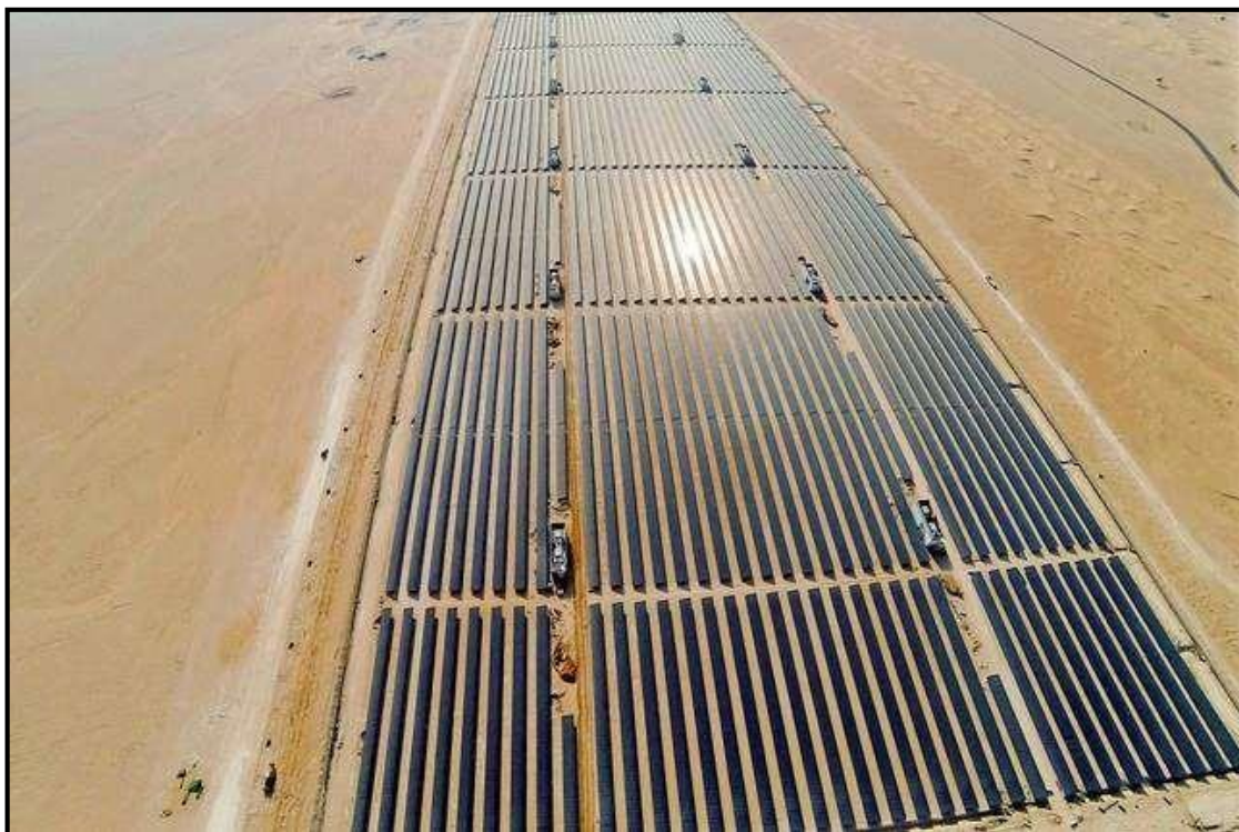
Figure 2: Typical Power Arrays Composed of PV Panels
