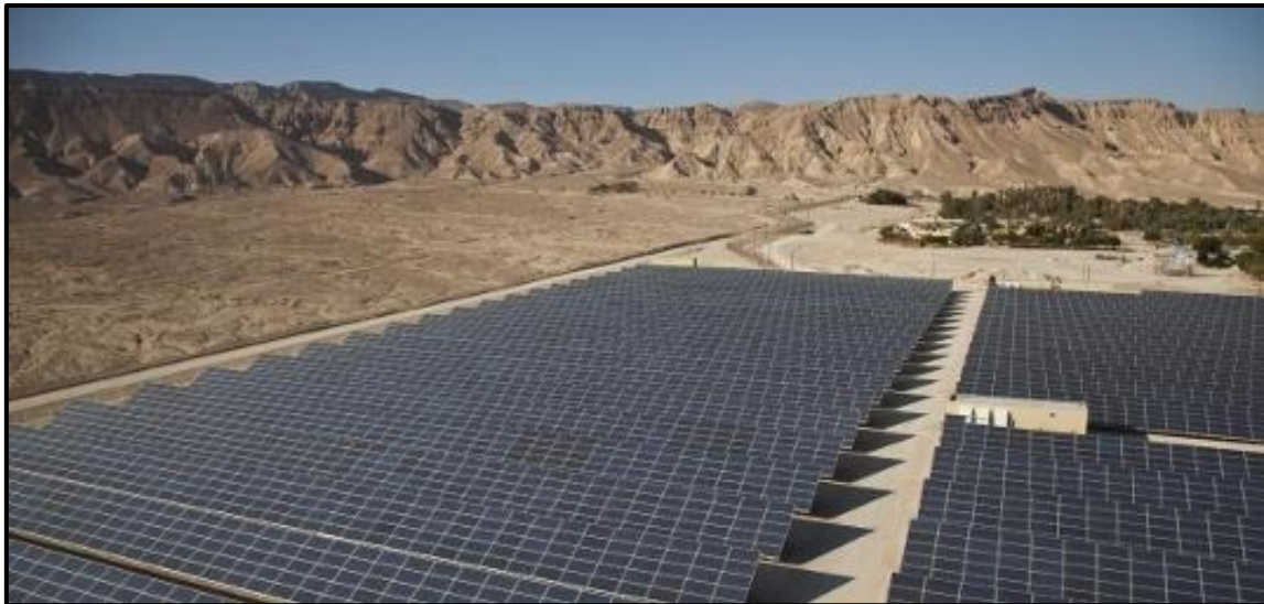
Figure 3: Typical Power Arrays Composed of PV Panels
