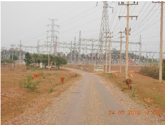
Plate 5-9 Hin Heup Substation, adjacent to Mill site
