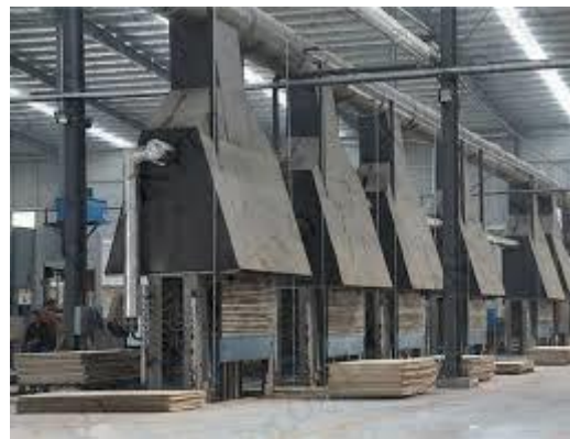
Plate 3-9 Plywood presses with ventilation
