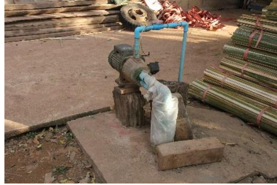
Plate 6-13 Water pump in Ban Houay Deua, Phonehong District
