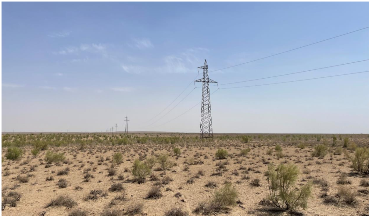
Plate 14-2 Existing Overhead Transmission Lines
