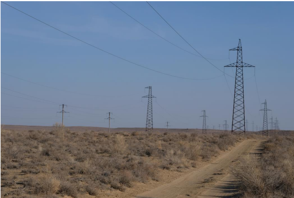
Plate 12-3 OHTLs in the Project Site
