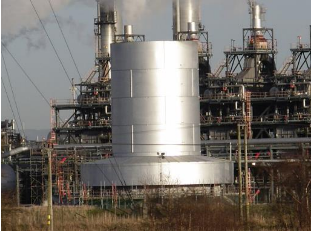
Figure 3-4: Typical Enclosed Ground Flare
