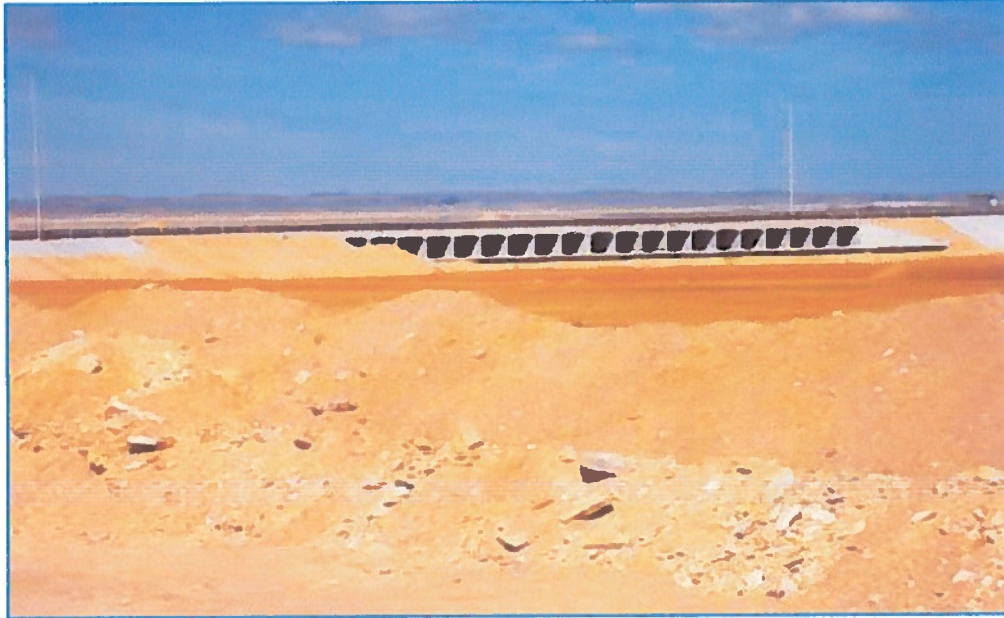
Figure (6. 25): One of drainage hydraulic structures at Wadi crossing road (Photo taken by K& A, 12- 2014)
