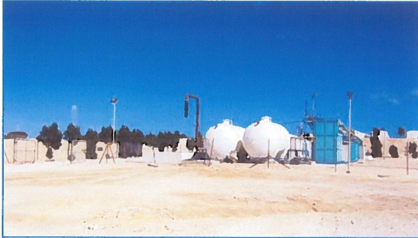
Figure (5. 2): Compact STP for manpower during construction (STRABAG contractor) (Photo taken by K&A, 12-2014)
