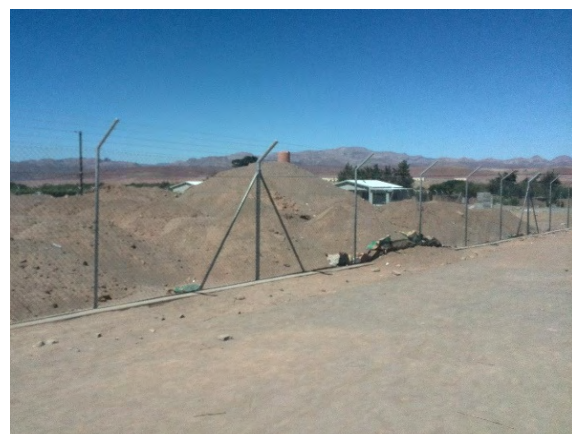
Photo 16. Construction Site of the Wastewater Treatment Works, View From Outside The Construction Perimeter
