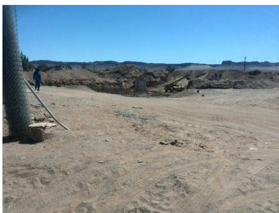
Photo 15. Construction Site of the Wastewater Treatment Works, View From Within the Construction Perimeter
